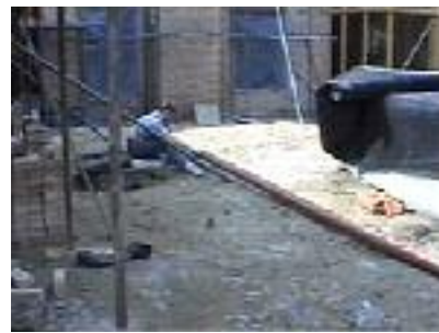
The sump at the rear needs pumping out
