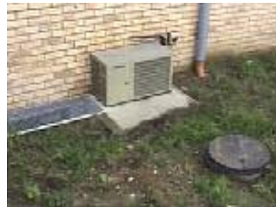
A chiller unit to cool the air on hot days.
