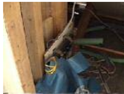
The pipework is still ...
