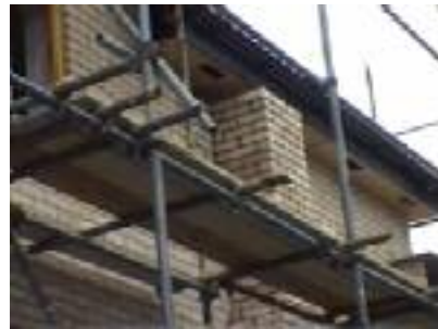
The chimmies would both need cutting through
