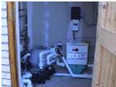
The swimming pool plant room.
