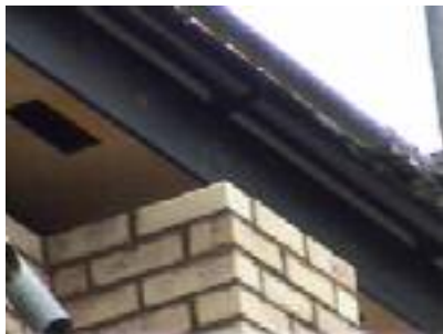
The gutter was in for a shock
