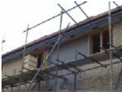
Someone put the air vents in a dum place!
