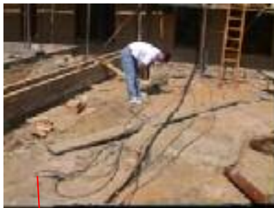
There was so much TV cabling it had to go outside!
