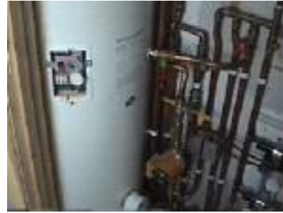
Hot water tank and plumbing
